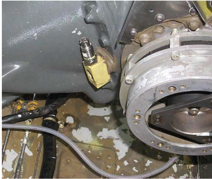
Figure 20. No. 2 Input Module Accelerometer Installation (ACC2)
